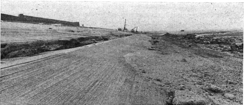
Fig. 11. New toe construction completed before start of facing reconstruction, showing sand accretion
