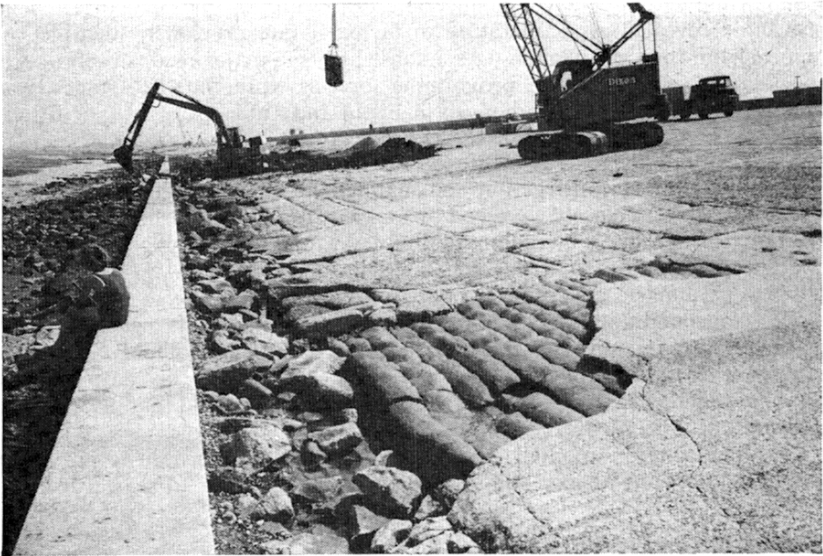
Fig. 9. Deteriorated facing prior to reconstruction, 1974: new precast toe beam in position
