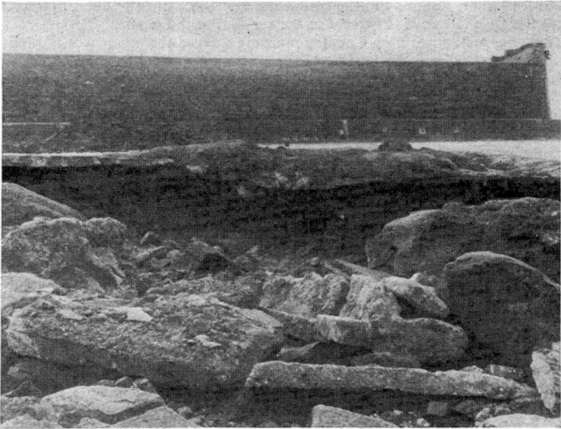
Fig. 15. Part of the deep break in November 1973 showing old 'non-tidal' facing concrete undercut by wave action
