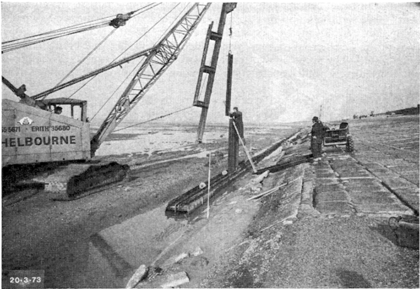
Fig. 10. New toe sheet piling being driven to seaward of old toe construction
